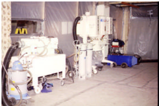
Figure 20: Off-board equipment setup
